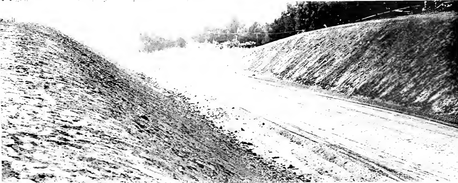
Top—Rough graded section of realignment of Coast Highway west of Santa Barbara. Center—Cut slopes being rounded preparatory to application of top soil. Bottom—Top soil applied and left rough to permit natural vegetation to gain a foothold
